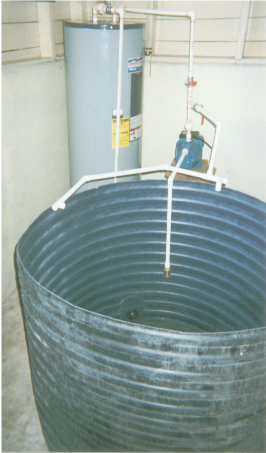
Figure 7. Front view (without water) of hot water treatment unit at the NGMC packinghouse. Note: plumbing of PVC pipe inside the tank is not completed.
